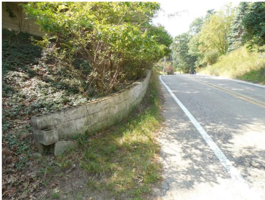
Photo 40: Existing masonry (CMU) retaining wall south of 405 Park Street, ~1' clear from edge of asphalt
