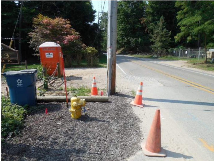
Photo 45: Utility pole at 183 Park Street, 2' clear to edge of asphalt
