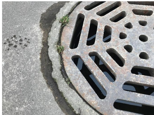
Figure 13 – Water level just below the frame
