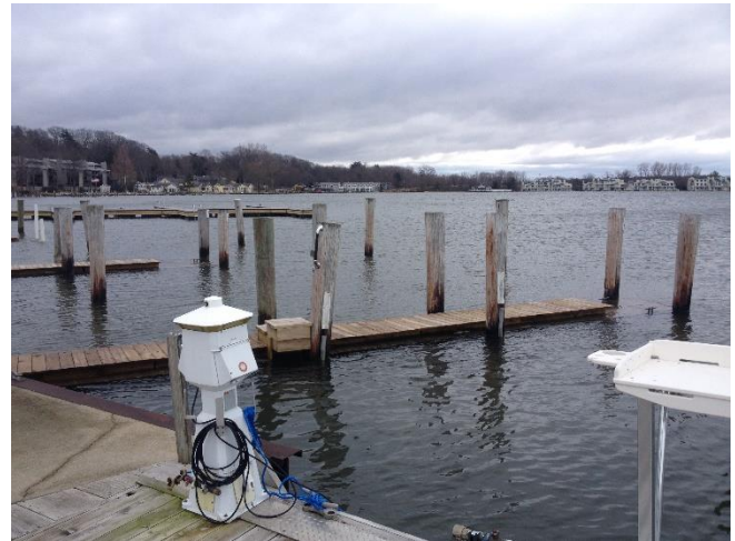
Figure 2 - March 6, 2020 Lower dock submerged
