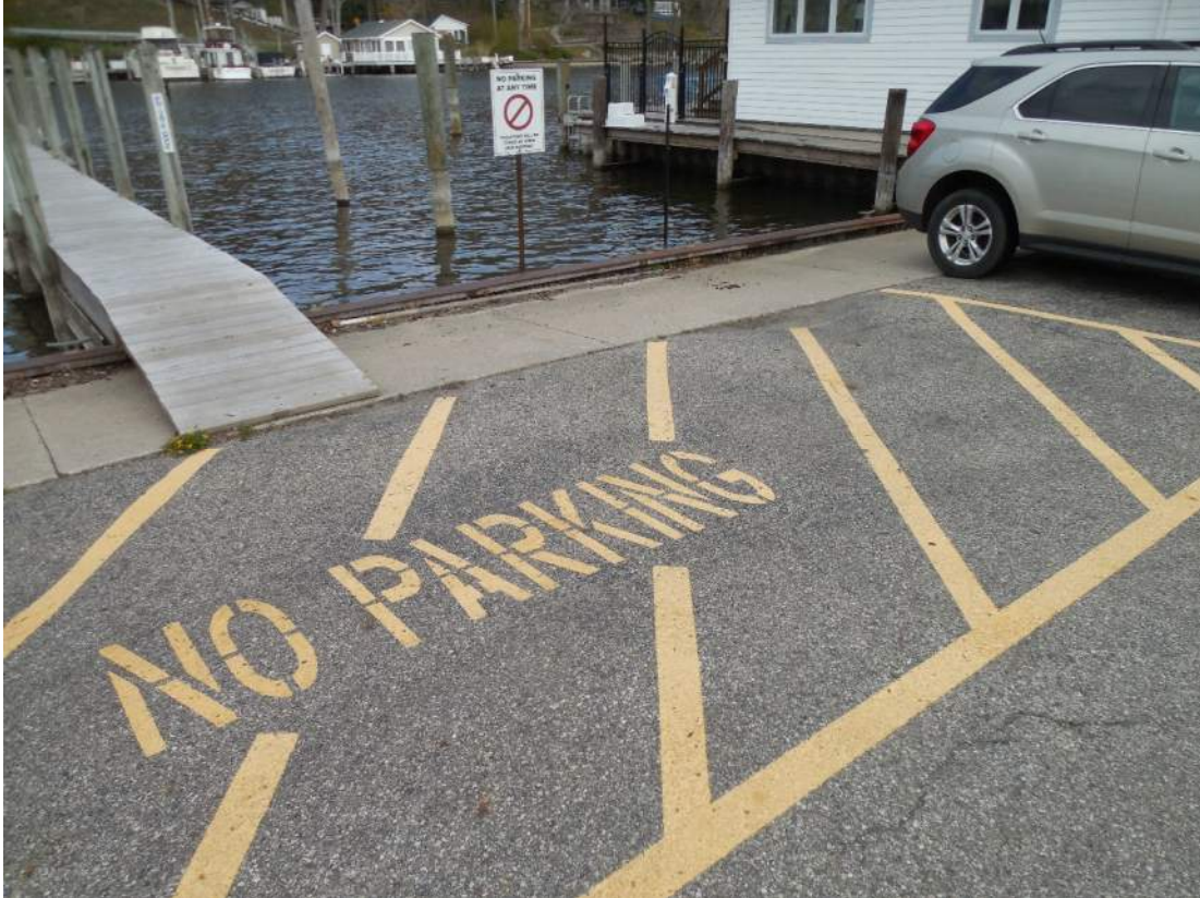
Settlement of Francis Street roadway along sea wall from high lake level and surface runoff
