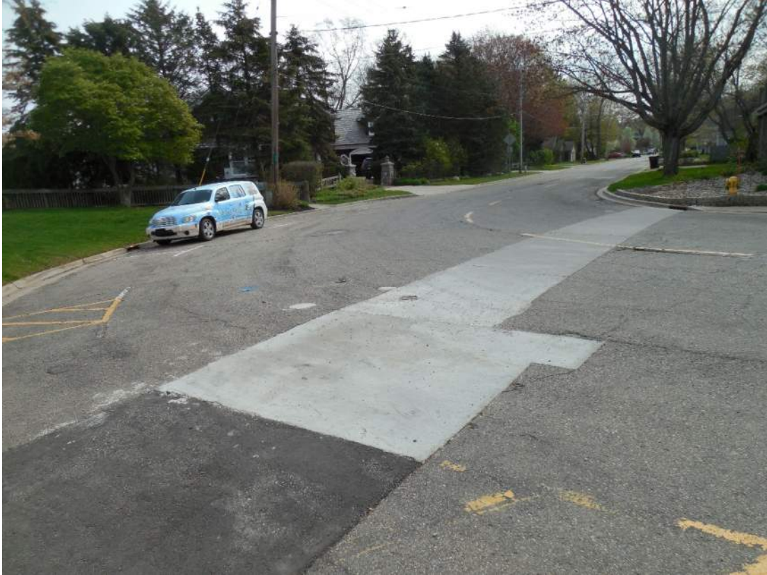
Patching from flooding mitigation measures at the intersection of Lucy and Water Streets
